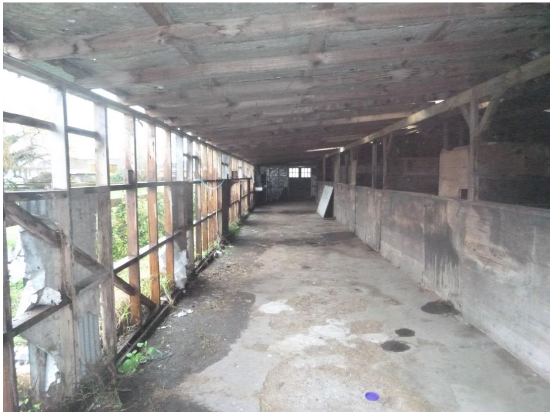
Photograph 3: Interior of Stable 2 (looking south). Note partially demolished wall on left of photo.
