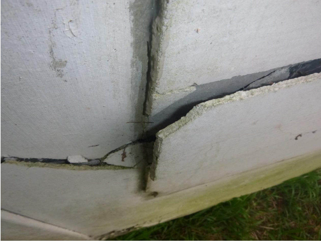
Photograph 4: Potential asbestos containing material (fibrecement cladding) found on Stable 2.
