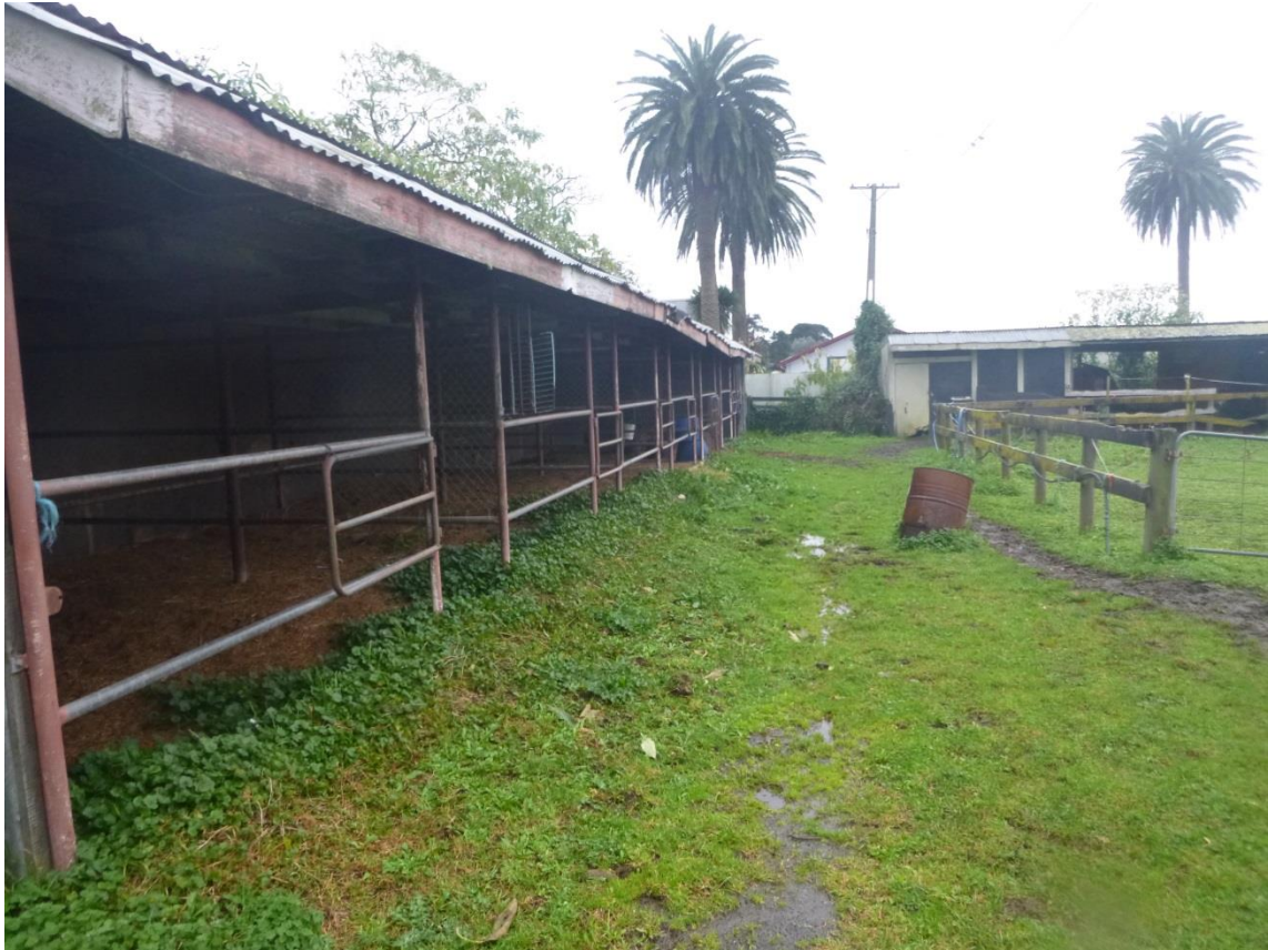
Photograph 6: Stables 3 and 4, note soil tracks cut by horse movements (looking north).
